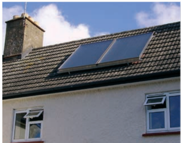
Solar water heating panels
